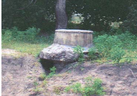
A borehole that served the clinic has lost its function
