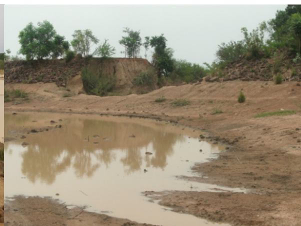
Plate 6: Broken Dam Wall at Piina
