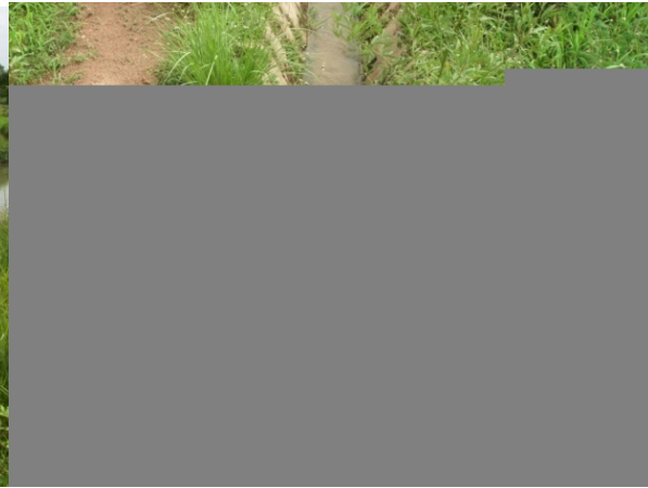
Plate 2: Dilapidated Canal at Bullu
