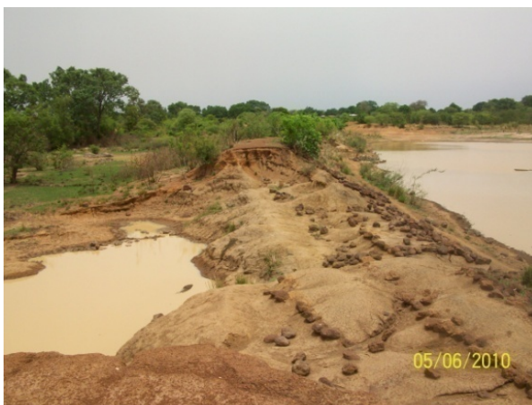
Plate 5: Broken Dam Wall at Piina
