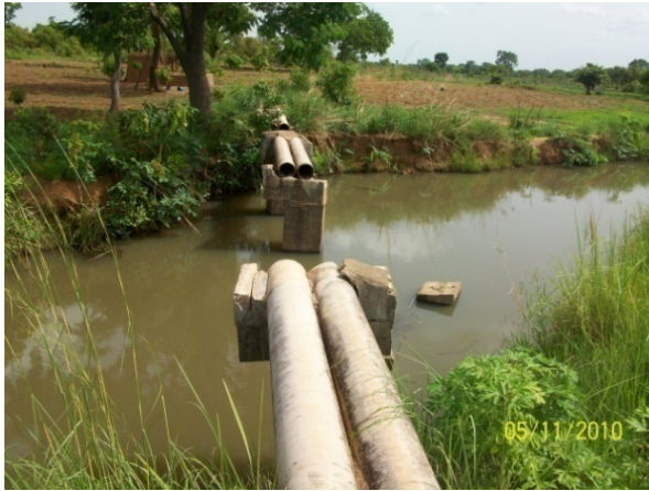
Plate 1: Broken Canal at Sankana Dam
