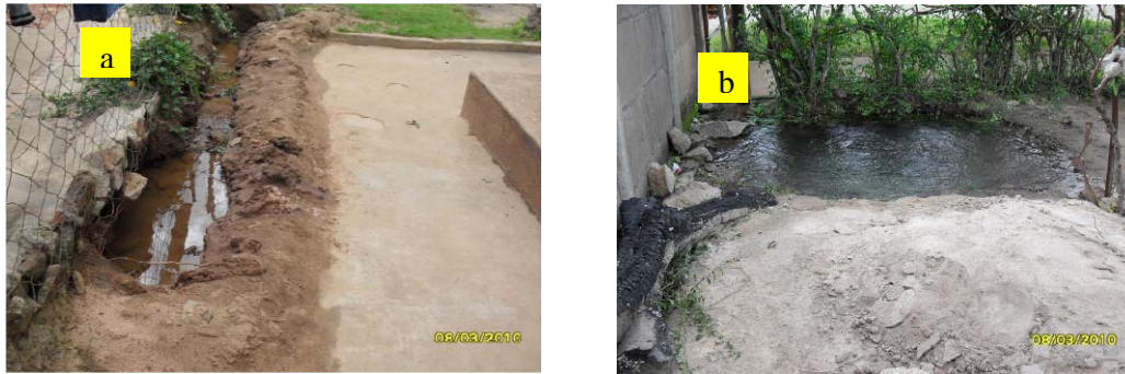
Figure 5: Water Loss from Pipe Bursts in the Residential Areas
