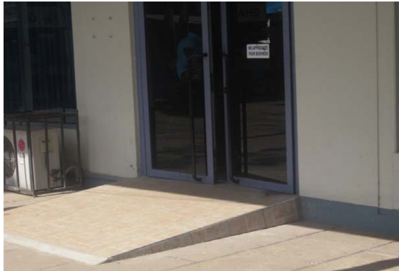
Figure 4: Ramp running directly to threshold of door with no landing
