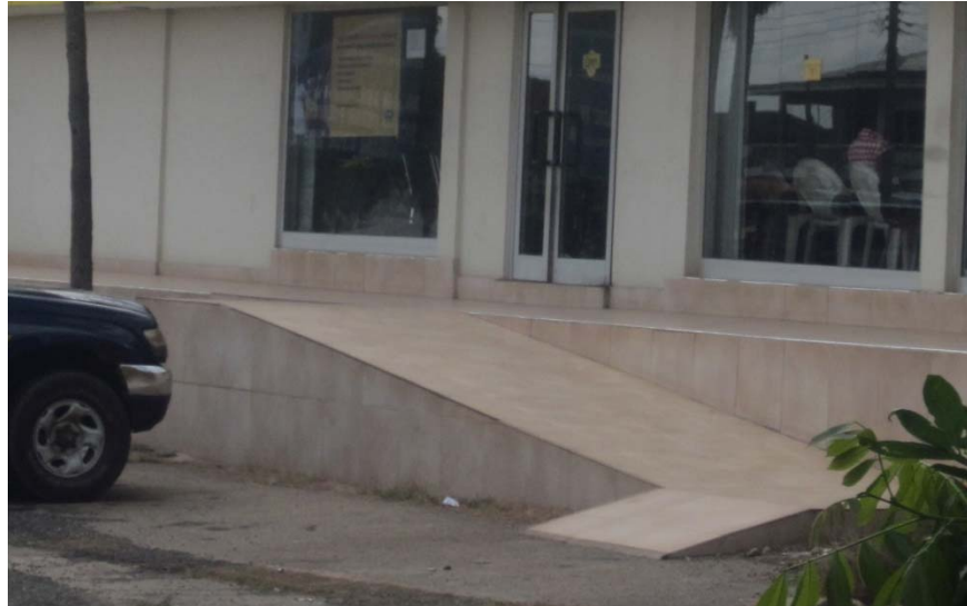
Figure 5: Ramp with no guiding handrails for users
