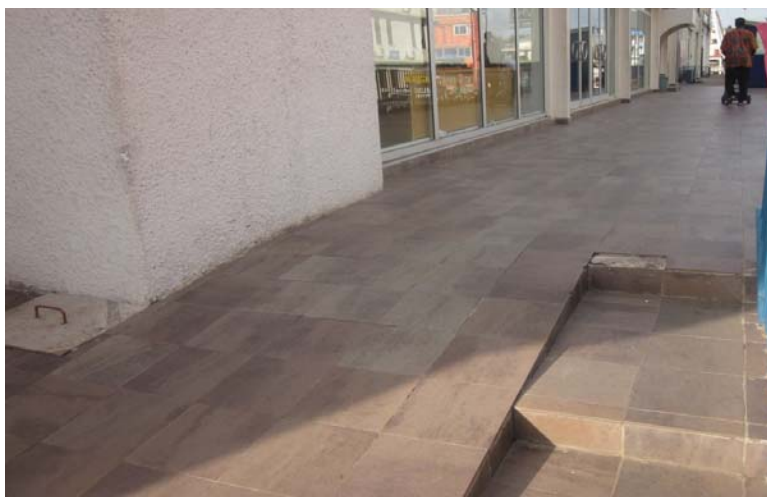
Figure 3: High thresholds at a main entrance doorway
